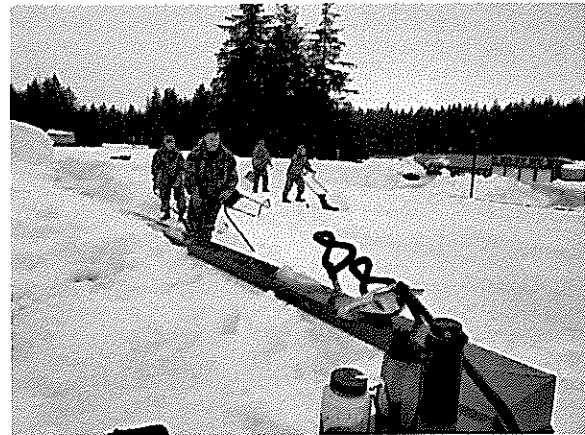
Snow removal at Elementary School, south side of building. 4 feet of depth was measured.
