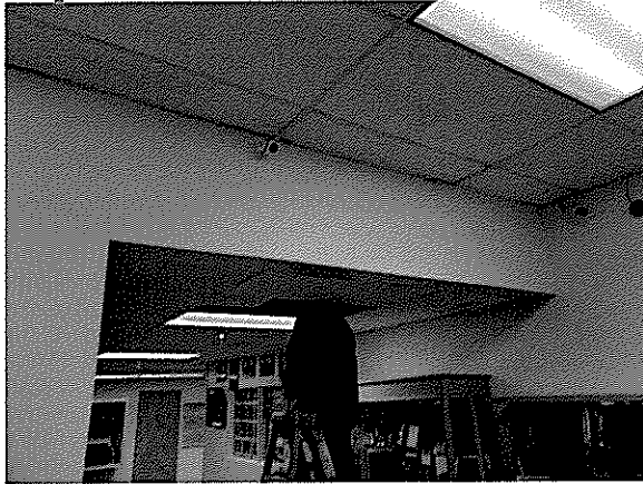
Ceiling transition at High School Lobby/Corridor has cracks on each end: Roof trusses are not supported by this but when they are moderately loaded the trusses push this 2x framed box beam down and the gypsum wall board cracks
