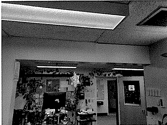
False Header in Receptionist Office: Not a structural member and can be removed. This is pushed down when roof trusses are moderately loaded
